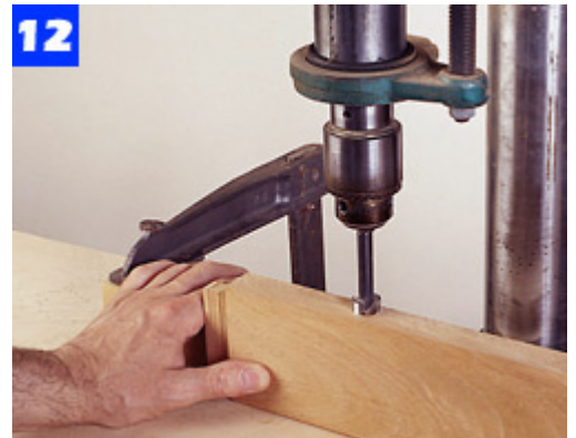
12 Clamp a fence to the drill press table to help position the aprons when cutting the tabletop fastener mortises.
