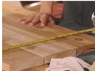
Measure the width of the bottom boards and cut a side board to fit.
