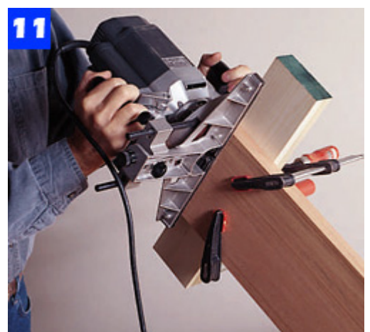
To rout the hanger mortises, clamp a board to the rail for router support. Use a small chisel to cut the deeper recesses.
