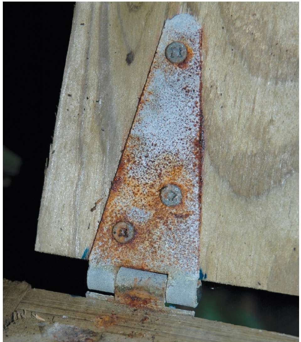
Corrosion of galvanized steel hinge attached to ACQ-treated wood. New preservative formulations can be very corrosive to metal. It is important to use the recommended fasteners when building a deck.
