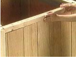
Cut the doors to fit inside the trim and one half to one inch off the ground
