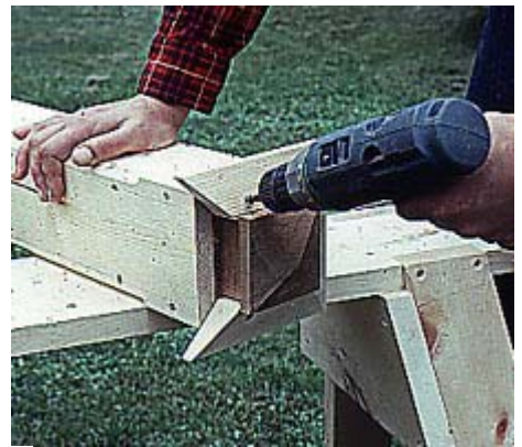
8--Slide three-sided collar around block from open side of post. Secure with screws and attach remaining side with glue and screws.
