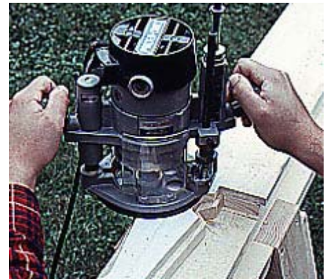
3--Use a router, 1/2-in. bit, 1-in. guide bushing and picket jig to trim the rough pickets to the finished shape.
