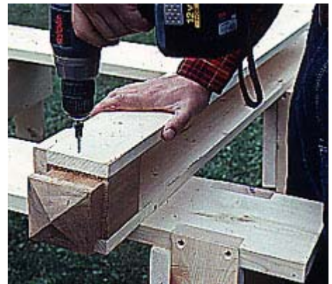
7--After routing the recess around each block, install three-sided posts and secure with a screw on two adjacent sides.
