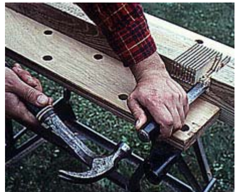
10--Cut 4 x 4 post notches by making a series of kerfs with a circular saw. Then remove the waste with a sharp chisel.
