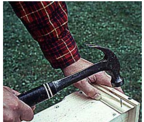
9--Use galvanized finishing nails to secure trim under the post collar around three sides of the box post. Drive two nails per piece.
