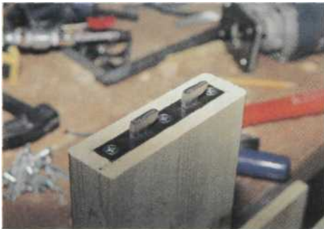
13 The knock-down hardware installed.
