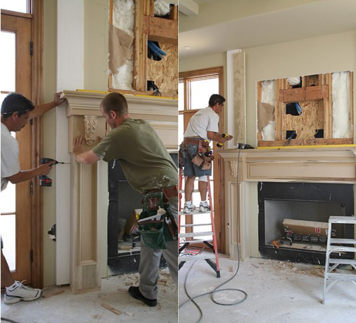
After fastening the lower mantel to the backing with trim-head screws, we attached backing to the pilasters for the upper mantel.
