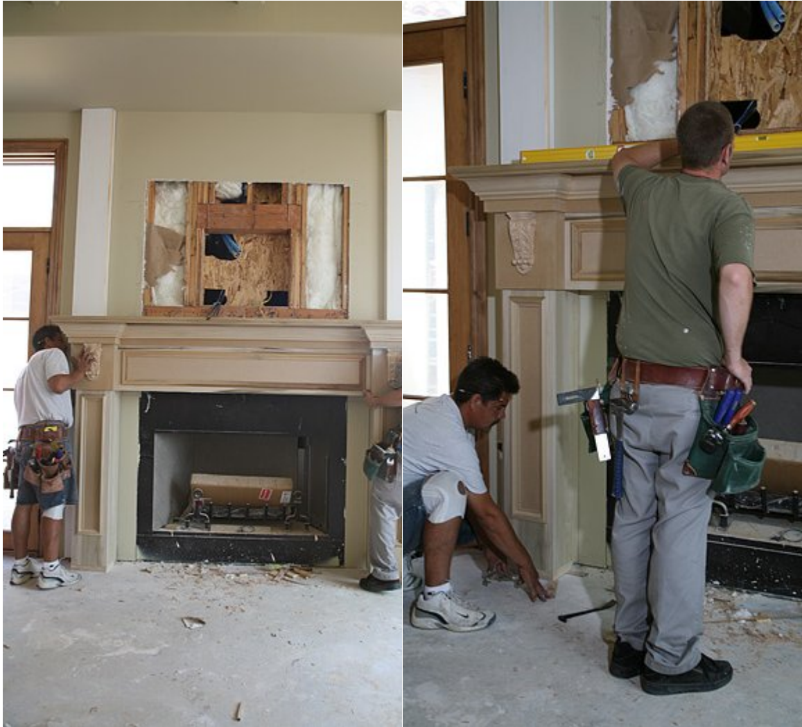
We slipped the pilasters over the backing, then shimmed the lower mantel level.
