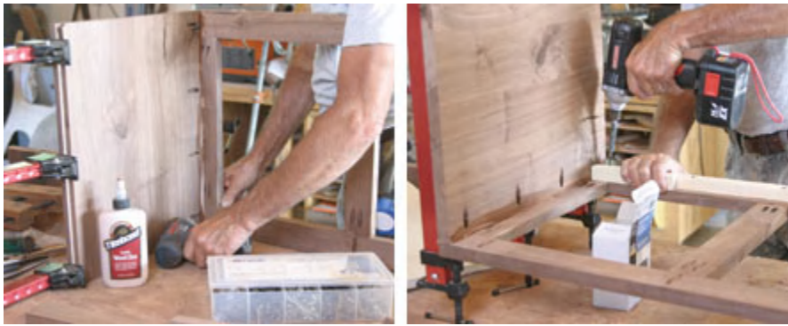
Left: Fasten the bottom section sides to the face frame with pocket-hole screws and glue. Right: Install bottom and top back supports. Fasten cleats on the inside of the case and install the bottom.
